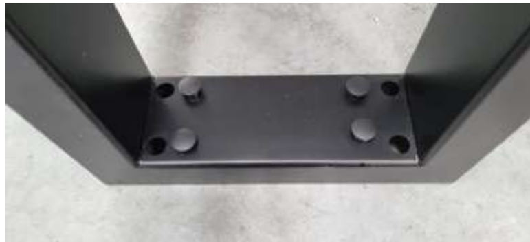
Base of steel frame where dyna bolts are Installed into the concrete floor. Also showing plastic covers
